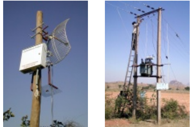
Fig. 3. Deployed sensors and GI poles
